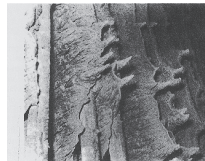
FIGURE 22-10 Precipitation fouling of ash particles on superheater tubes.
