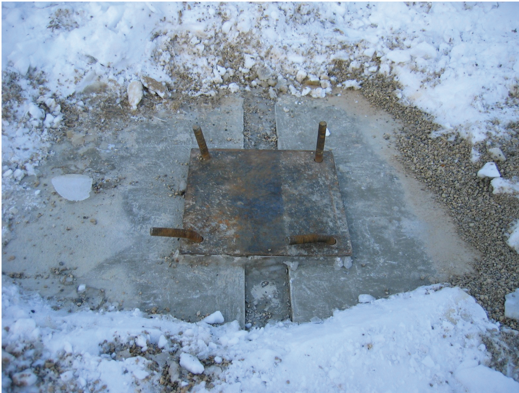
Fig. 4-17. Anchor rods run over by a crane.
