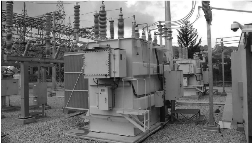
FIGURE 2.20 A distribution substation operating at a 34.5/4.16 kV voltage level. (Union Electric Company.)
