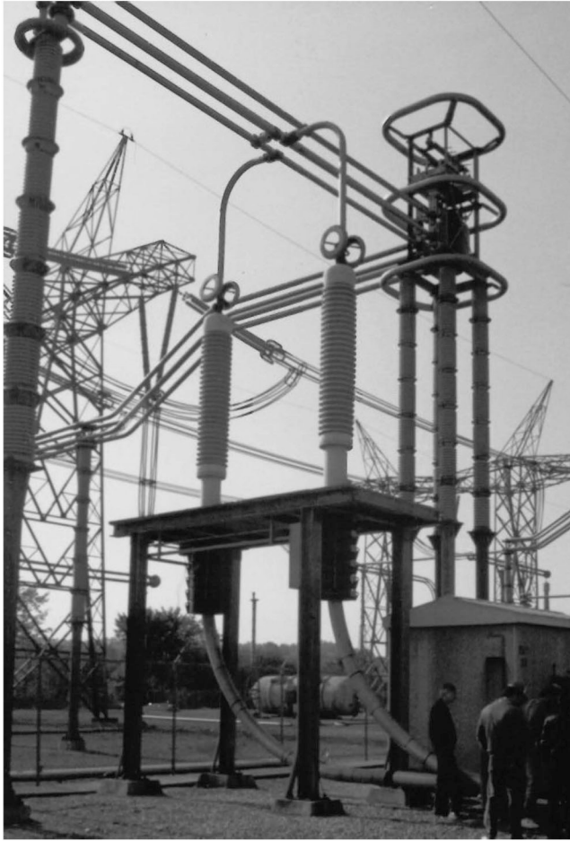
FIGURE 5.11 800 kV risers on the AC side at the same converter station.
