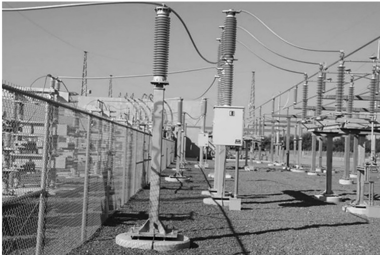
FIGURE 7.3 Single-pole-operated 138kV SF 6 live tank circuit breakers. (Courtesy ABB Corporation, Munich, Germany.)
