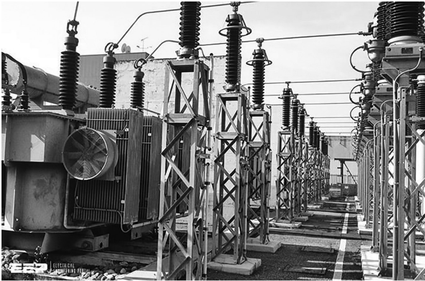
FIGURE 2.19 A distribution substation operating at a 34.5/12.47 kV voltage level. (Union Electric Company.)
