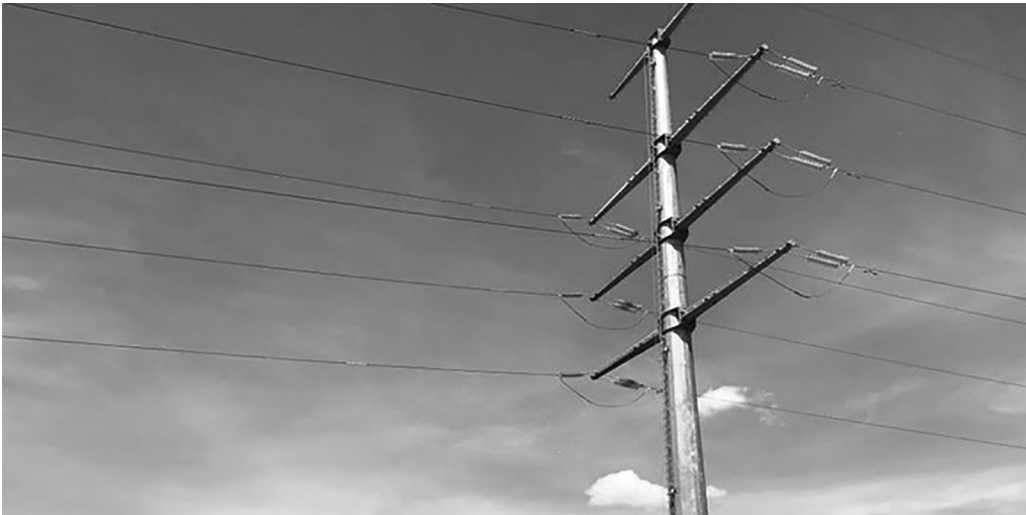
FIGURE 2.13 A typical 34.5 kV line with a double circuit and wood poles. It has a newer style construction. (Union Electric Company.)
