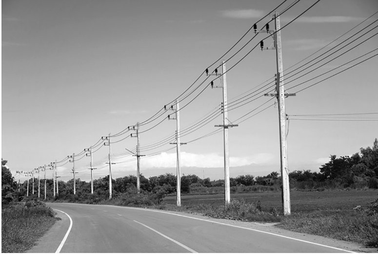
FIGURE 2.15 A typical 34.5kV line with a double circuit and wood poles. It also has a 4.16kV underbuilt line and a 34.5kV switch. (Union Electric Company.)
