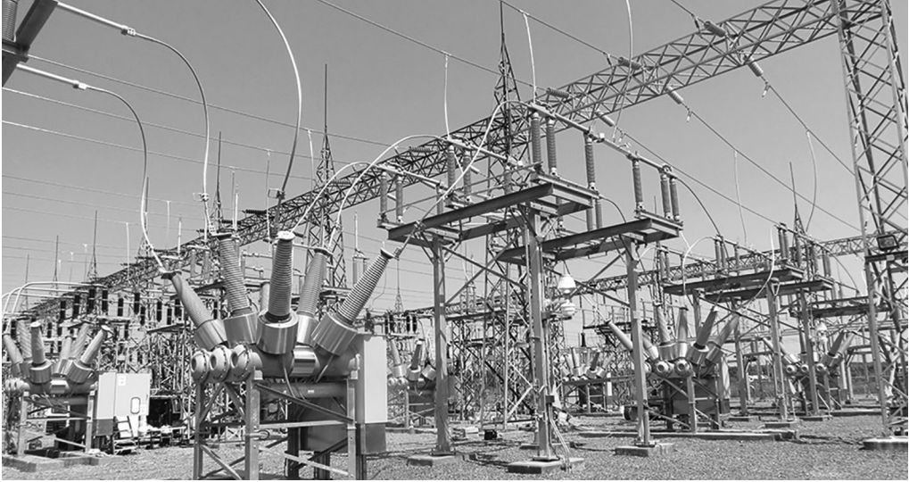
FIGURE 2.18 A bulk power substation operating at a 138/34.5 kV voltage level. (Union Electric Company.)
