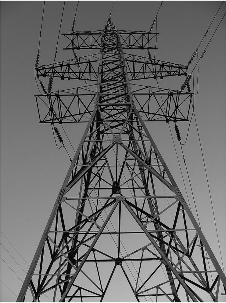
FIGURE 2.8 A typical 230kV transmission line steel tower with bundled conductors and double circuit.
