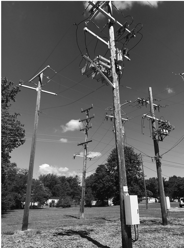
FIGURE 2.16 A typical 12.47kV line with a single circuit and wood pole. It has a newer type of pole-top construction. (Union Electric Company.)
