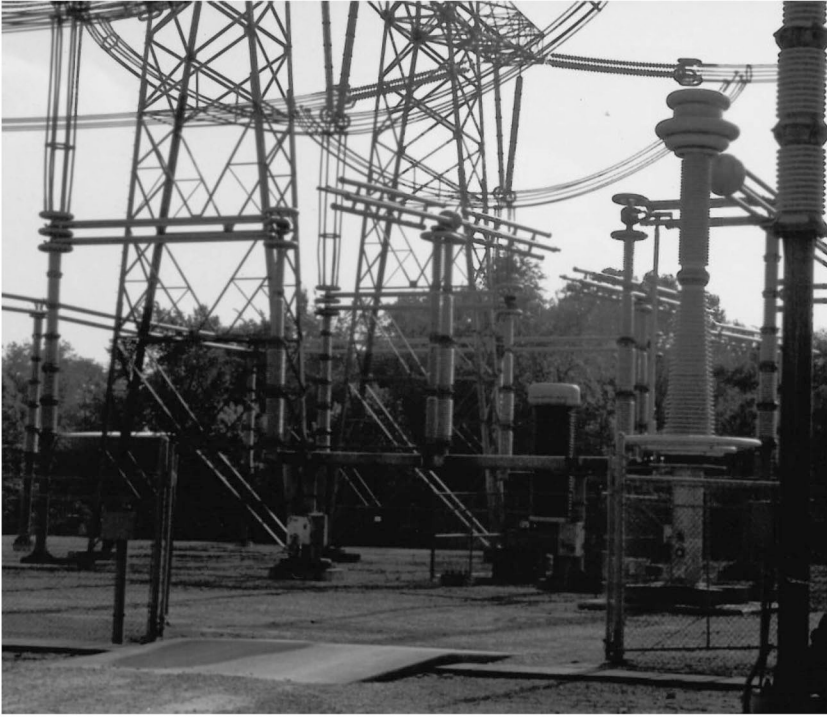
FIGURE 5.10 An 800 kV disconnect switch on the AC side at the same converter station.
