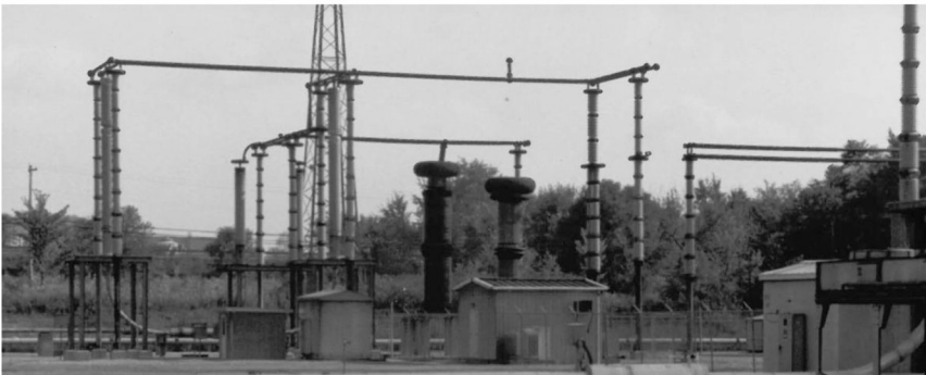
FIGURE 5.9 800 kV DC terminals of a converter station.
