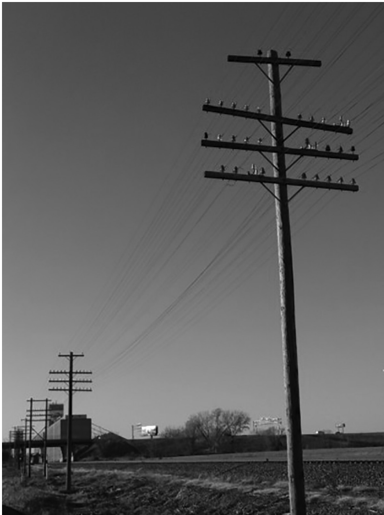
FIGURE 2.14 A 34.5 kV line with a single circuit and wood poles. It also has a 12.47 kV underbuilt line and 34.5 kV switch. It has an old style construction. (Union Electric Company.)
