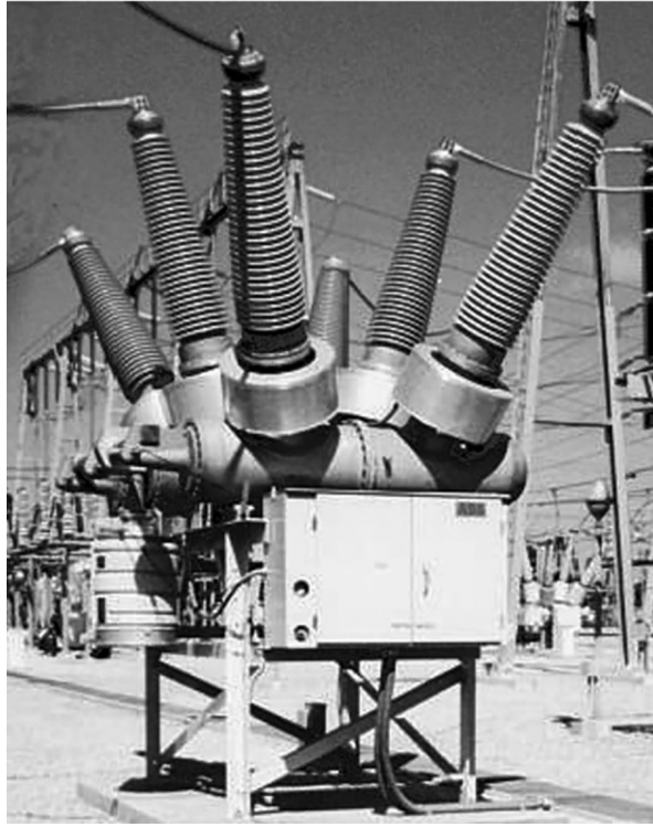
FIGURE 7.2 Three-pole-operated 245kV SF 6 dead tank circuit breaker fitted with 80 kA interrupters. (Courtesy ABB Corporation, Munich, Germany.)
