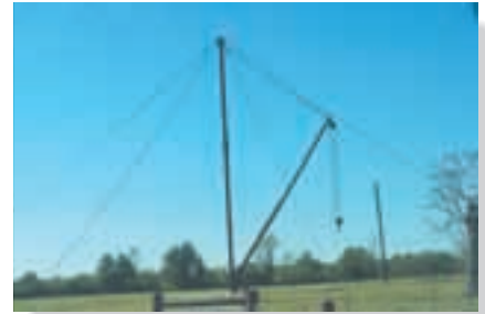
This crane is a typical example of a framework. (© Russell C. Hibbeler)
