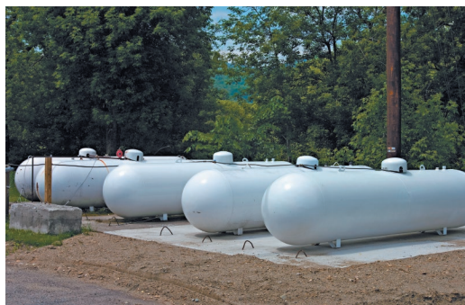
Photo 14.3 Cylindrical pressure vessels for liquid propane.
