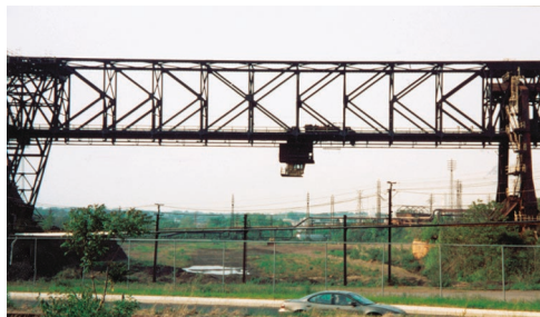
Photo 6.3 Two K trusses were used as the main components of the movable bridge shown, which moved above a large stockpile of ore. The bucket below the trusses picked up ore and redeposited it until the ore was thoroughly mixed. The ore was then sent to the mill for processing into steel.
