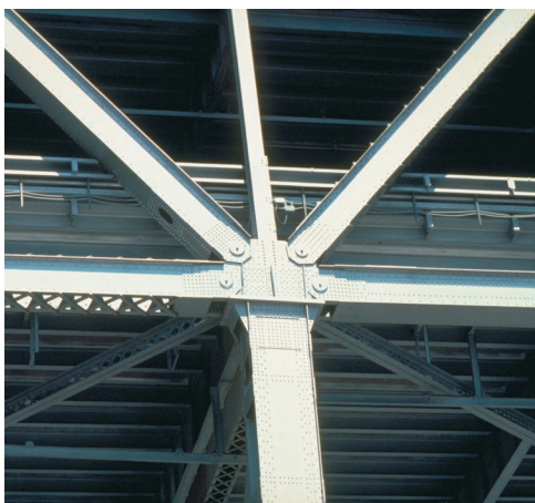
Photo 6.2 Shown is a pin-jointed connection on the former approach span to the San Francisco–Oakland Bay Bridge.
